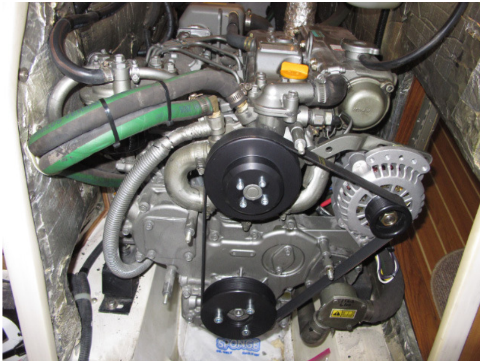
Electromaax PK-4JH4 + SM alternator all installed
